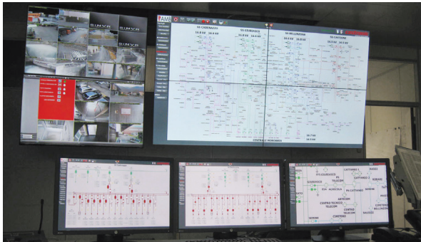
Figure 1: In the control room, the employees always have an overview of the complete energy grid and can zoom into the details at any time.
