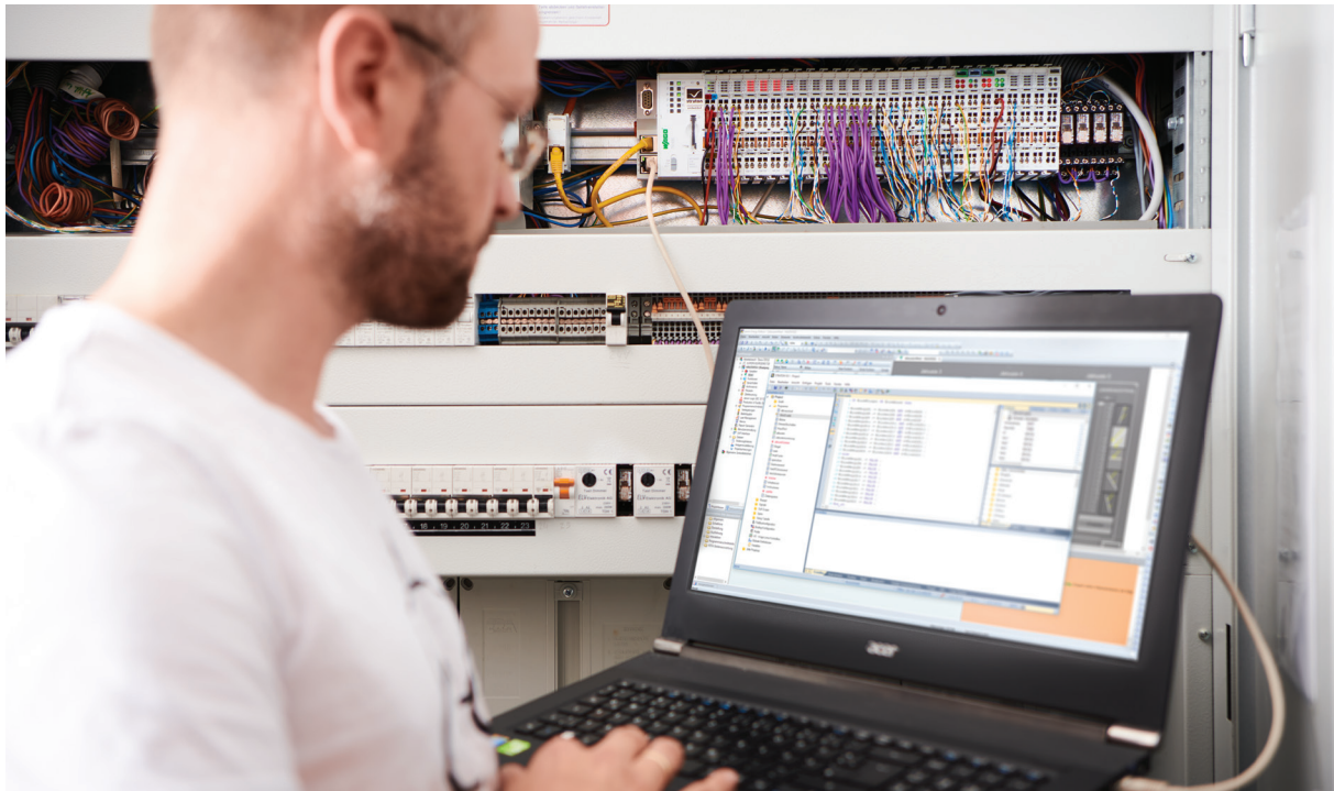
Markus Wintersteller configures his zenon project, which is connected to the central WAGO control system.
