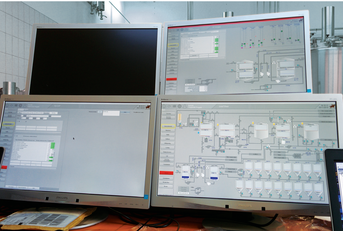
Figure 1: The master brewer can keep track of the entire production process at a glance via the multiple monitors displaying supervision application information in the control room.
