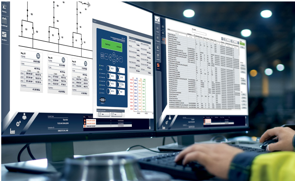
Figure 1: All information is collected in a substation HMI for a perfect overview.
