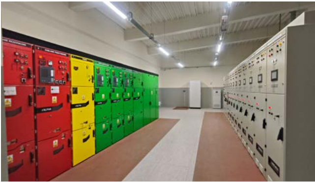
Medium voltage and direct current switchboards in a tram traction substation.
